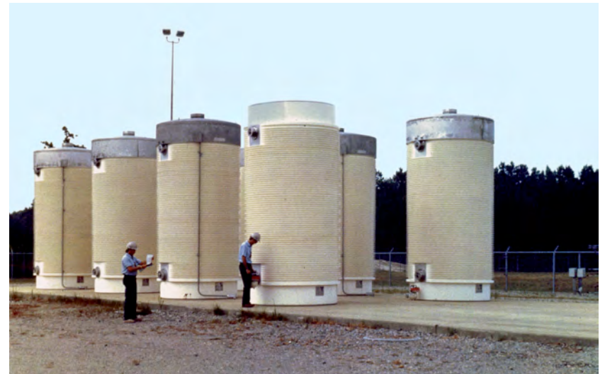
Dry Cask Storage
